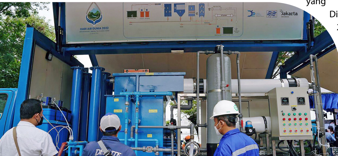
Gambar II.3. Mobil Pengolahan Air PAM Jaya
