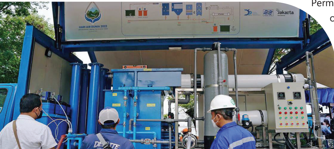
Gambar II.3. Mobil Pengolahan Air PAM Jaya
